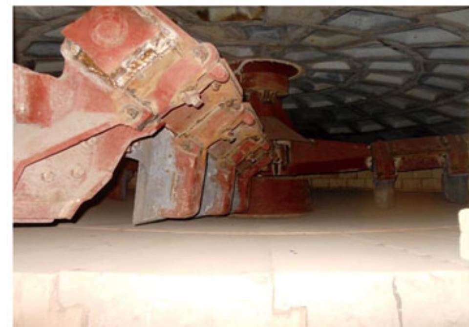
炉内件 Furnace inner parts
